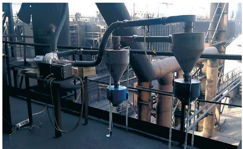
Portable pilot dust cleaning unit with a capacity of 200 m 3 /hr.
