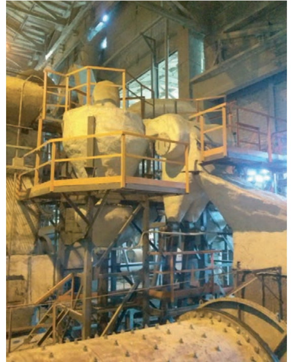
Photo. Centrifugal filters in the cement grinding mill gas cleaning system No.10 – 3,2*15, Balakleisk Cement Plant
