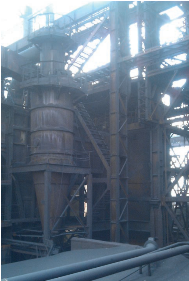
Upgraded L4H-15 cyclone for the dry coke quenching plant
