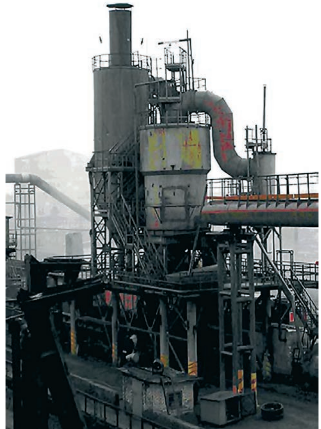
Upgraded gas filtering scrubber for the coke furnace battery
